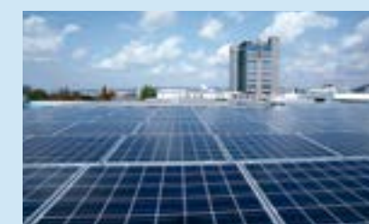
Introduction of solar power generation equipment: Group total output 2,180kW
